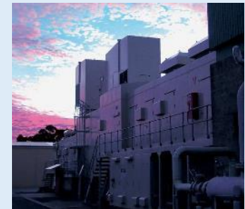
Synergen Power peaking station, SA (396MW)
