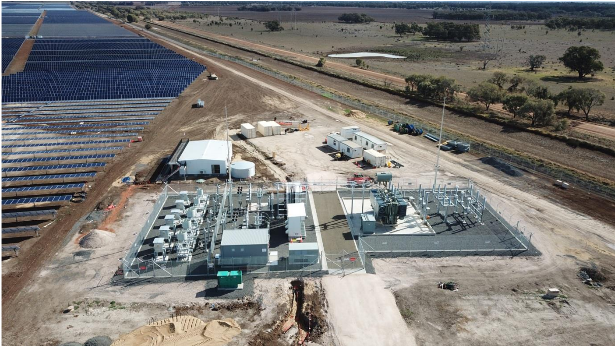
Plate 15 Example Terminal Substation (Colleambally Solar Farm)
