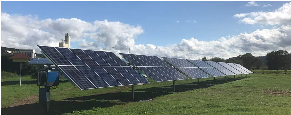
Plate 11 Typical Single Axis Tracking System
